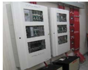
Fire Alarm System
