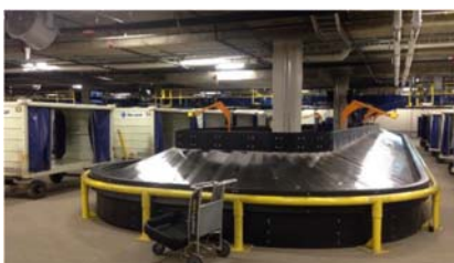
Baggage Handling System
