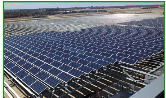
In 2014, the MAC and Ameresco Announce the World's Largest Structure-Mounted Solar Power Installation, Which is Constructed Atop MSP Parking Ramps
