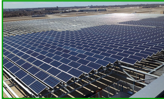
In 2014, the MAC and Ameresco Announce what was then the World's Largest Structure-Mounted Solar Power Installation, which is Constructed atop MSP Parking Ramps
