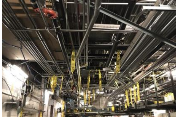
Baggage Handling System
