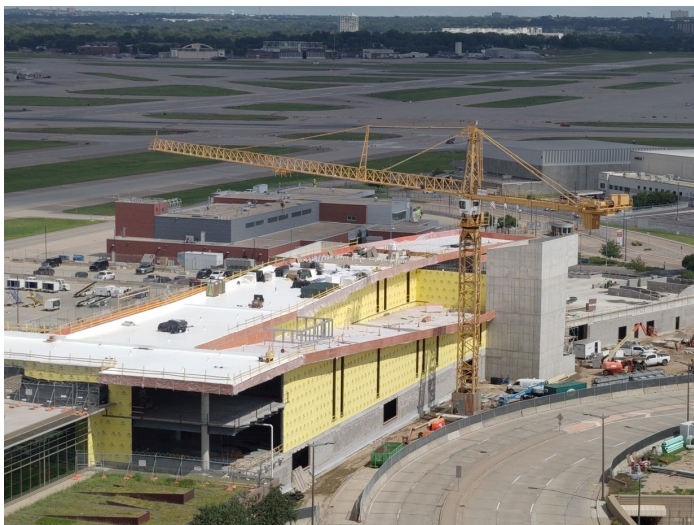
Construction of Two Additional Gates Including Gatehold Spaces, Expansion of Current Gatehold Spaces and Concessions at Terminal 2
