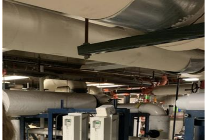
Victaulic Piping at Terminal 2
