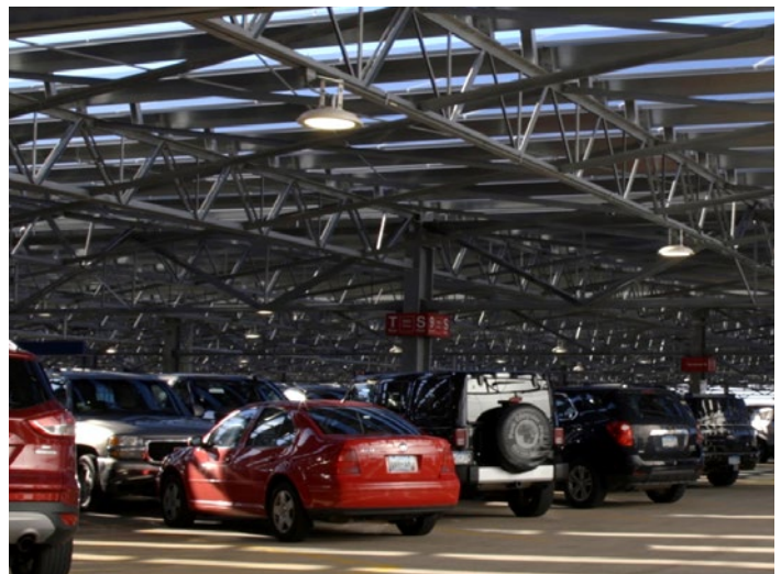
Energy-saving LED technology light fixtures in MSP parking ramps.
