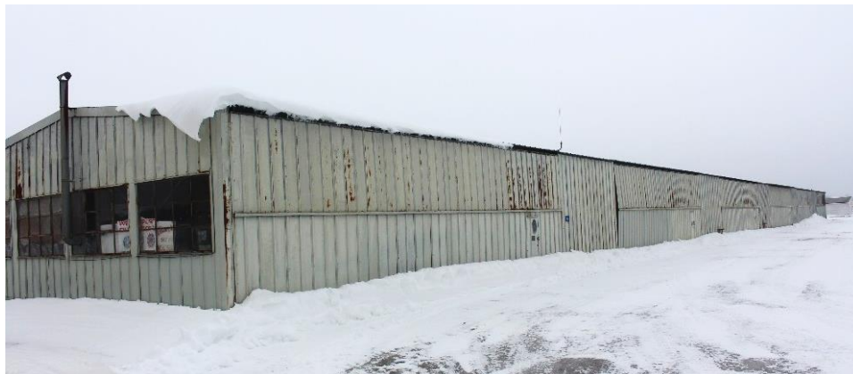
Figure 58. A ca. 1953, multi-unit T-hangar with five alternating stalls on each side in Hangar Area 1.
