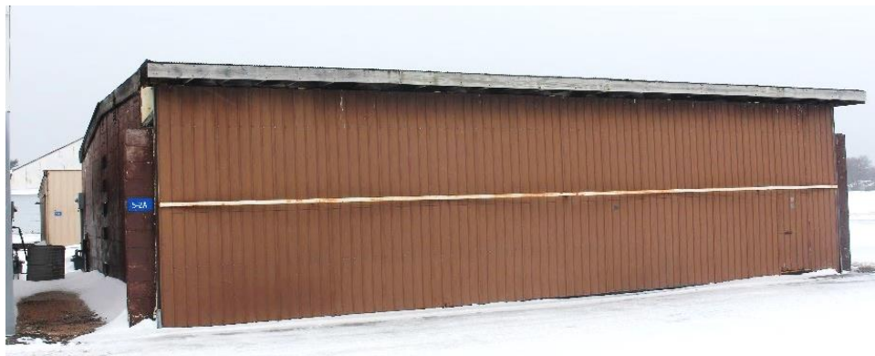
Figure 56. A ca. 1956 box hangar in Hangar Area 1. Note the concrete block wall and (likely replacement) bifold door.
