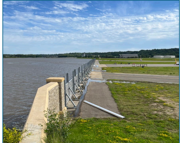
Floodwall deployed during active flood, July 2024 Source: Kimley-Horn
