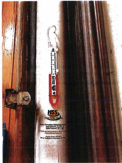
Vapor system monitor at building overlying source area, showing inactive pressure differential (currently unused port)
