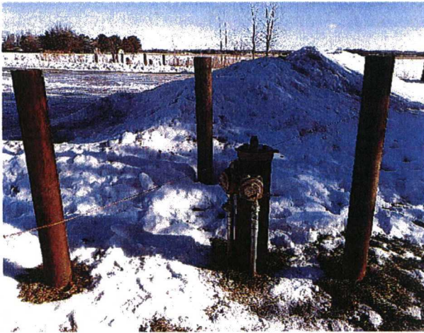
Source area extraction well (currently inactive to improve treatment effectiveness)
