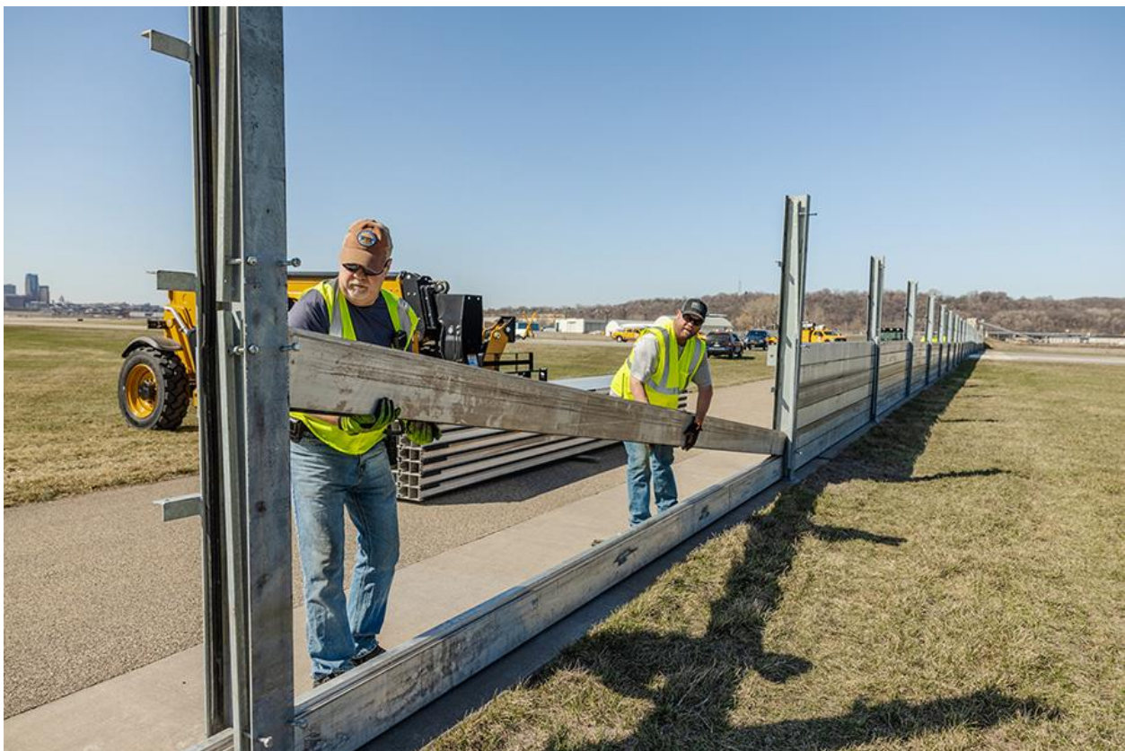
A MAC crew installs a section of the temporary floodwall at St. Paul Downtown Airport on April 13, 2023.
